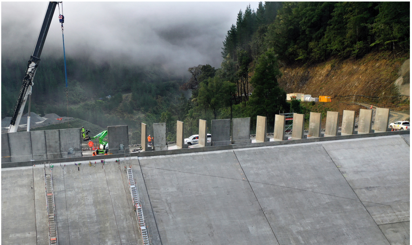
The installation of the parapet wall on the top of the Waimea Dam, forming a wave break.
